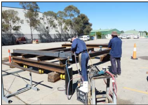
The installation process of the rock shovel bucket. Photo: Ainslie Greiner, National Museum of Australia.
